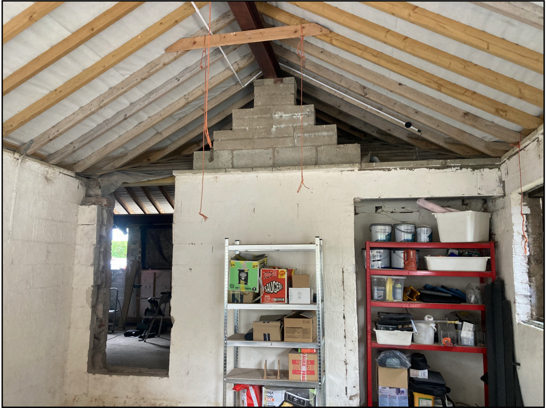
Figure 6: Internal space - this is from inside the byre and looking the barn section through the door - no potential voids internal and no wall top gaps or crevices suited to bats. NB. Nesting swallows were present to both the byre and the barn.
