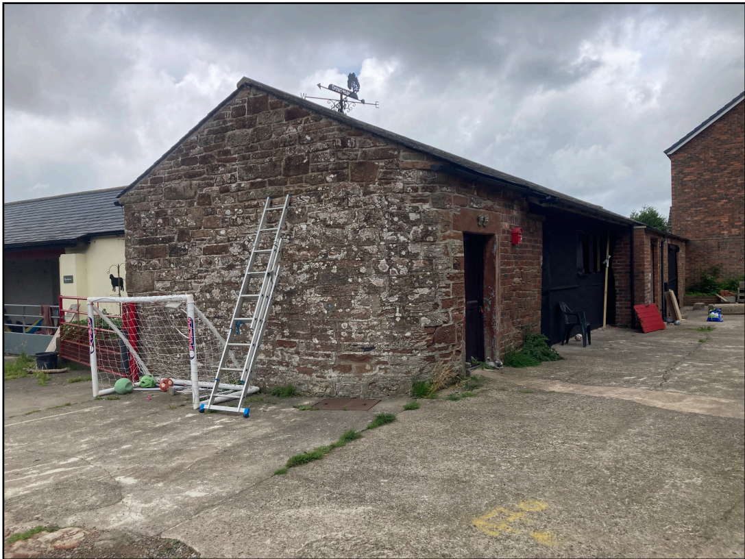
Figure 4: Showing the southwestern gable end - despite a through search of the entire buildings area, from ladder height there was no typically suitable access for bats present. To the left is the small section of byre which will provide utility space as shown in Figure 3.
