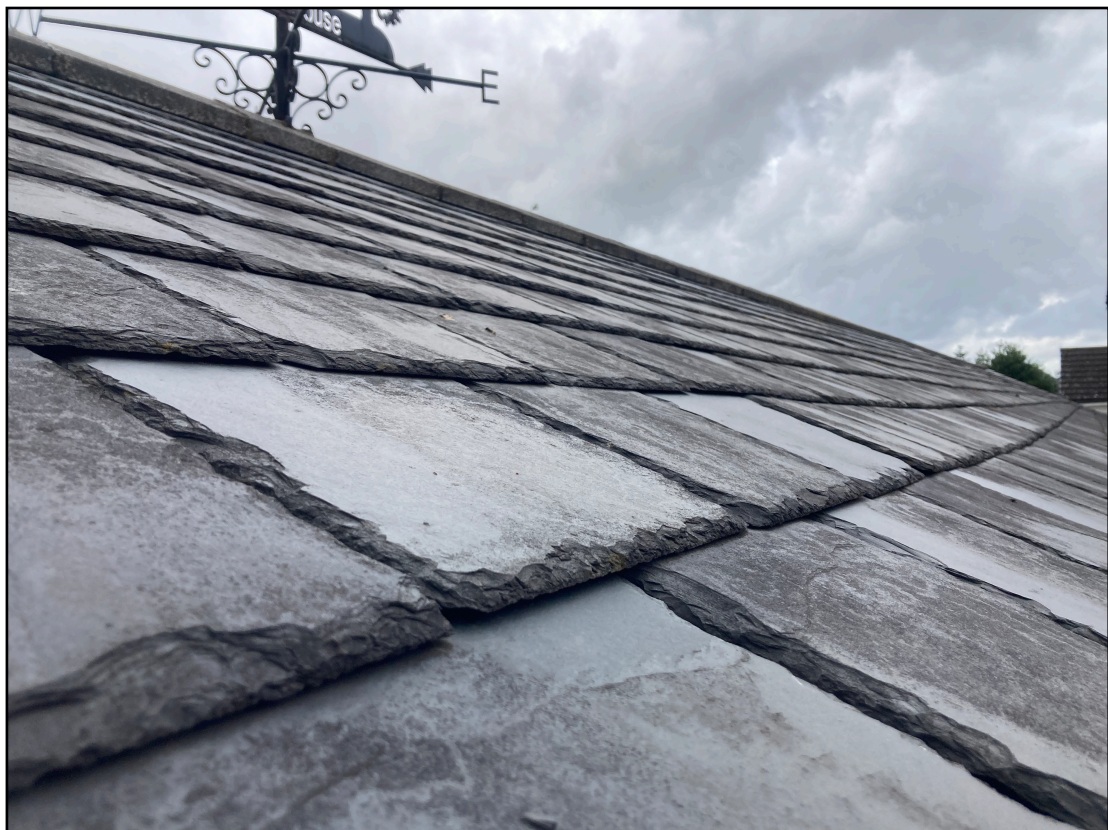
Figure 5: Showing the slate clad roof and cement ridges - very tightly set and no access for bats throughout.
