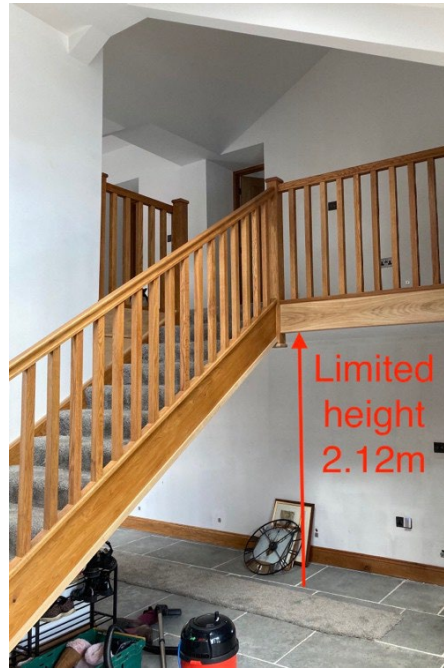
2 - Limited headroom under landing
