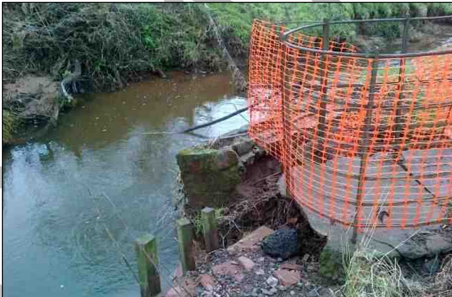
Photograph 2: Bank damage near the Sports Pitches (15 th December 2015)
