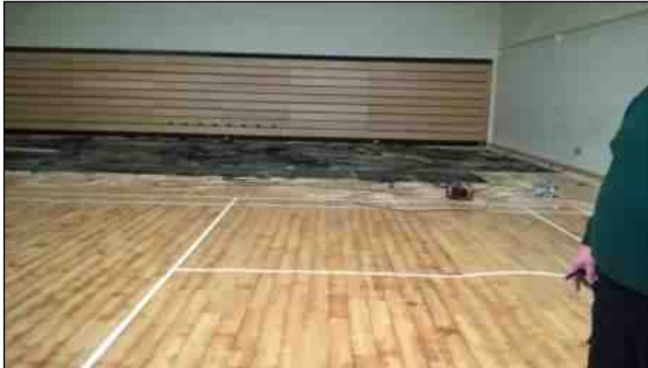
Photograph 9: Nelson Thomlinson School – Sports Hall Flood Damage
