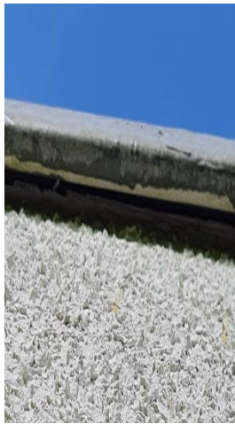
Photograph 1: Gap between wall and roof of garage
